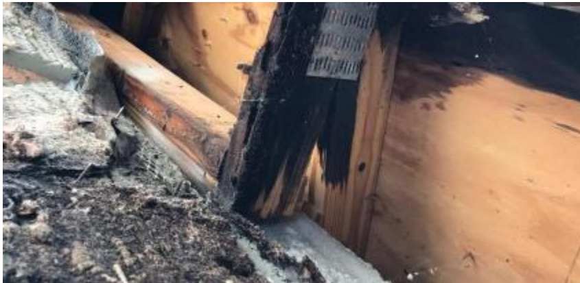
The San Matera Condominium Association presented this photo as evidence of construction defects at the Palm Beach Gardens property.
