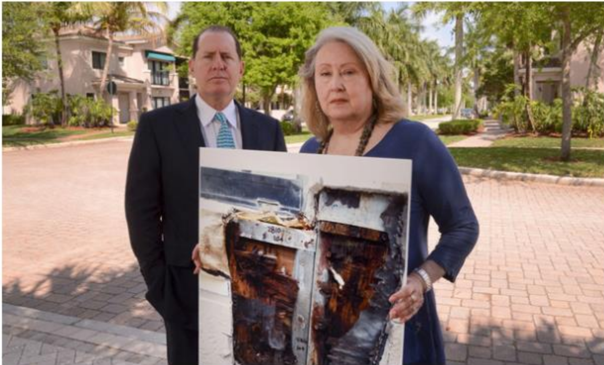
San Matero condo association's Jackie Durham holds an image of the the condition of the walls at a building there with attorney David Haber.
