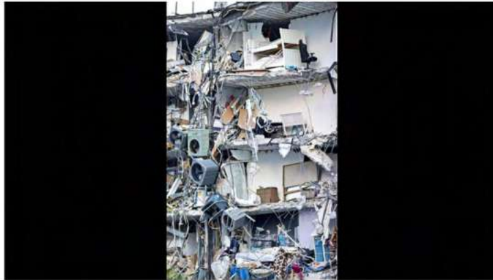
Mere feet separated the living from the dead when half of Champlain Towers South fell. The Herald has explored the structural roots of why and how it collapsed. David Santiago DSANTIAGO@MIAMIHERALD.COM
