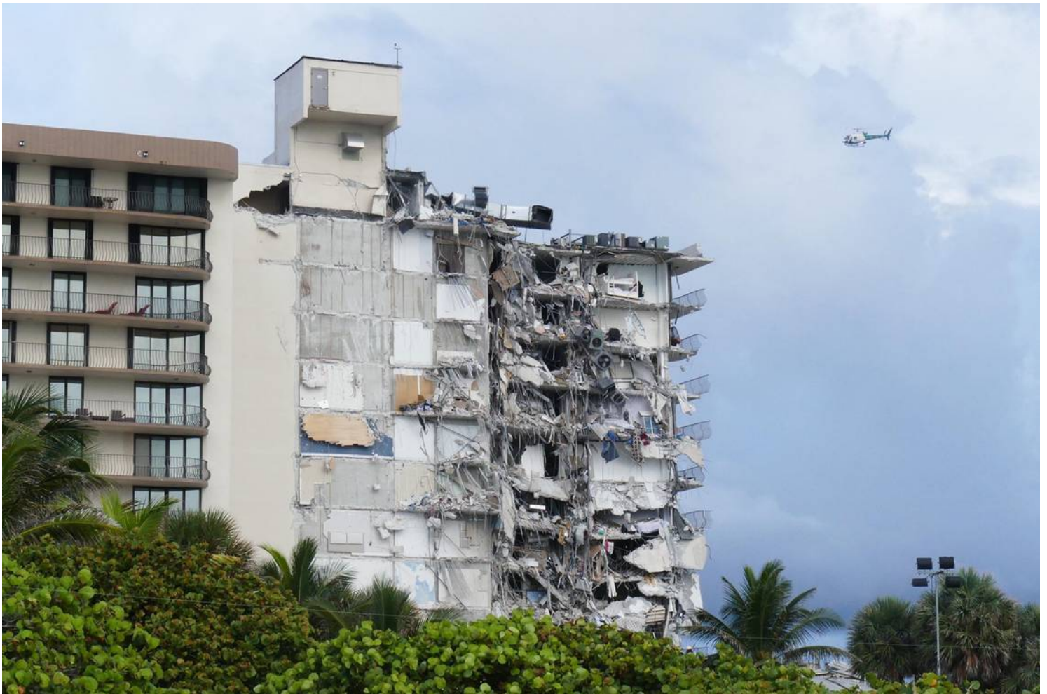
Florida lawmakers failed to pass legislation to address the most serious issues that emerged from the Champlain Towers South collapse in Surfside. Miami Herald
