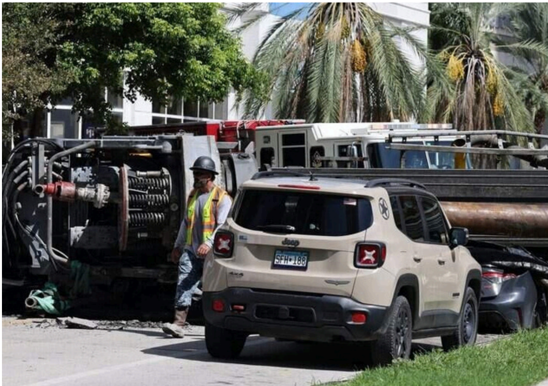
Construction equipment fell onto several cars on Brickell Bay Drive on Monday morning. Carl Juste cjuste@miamiherald
